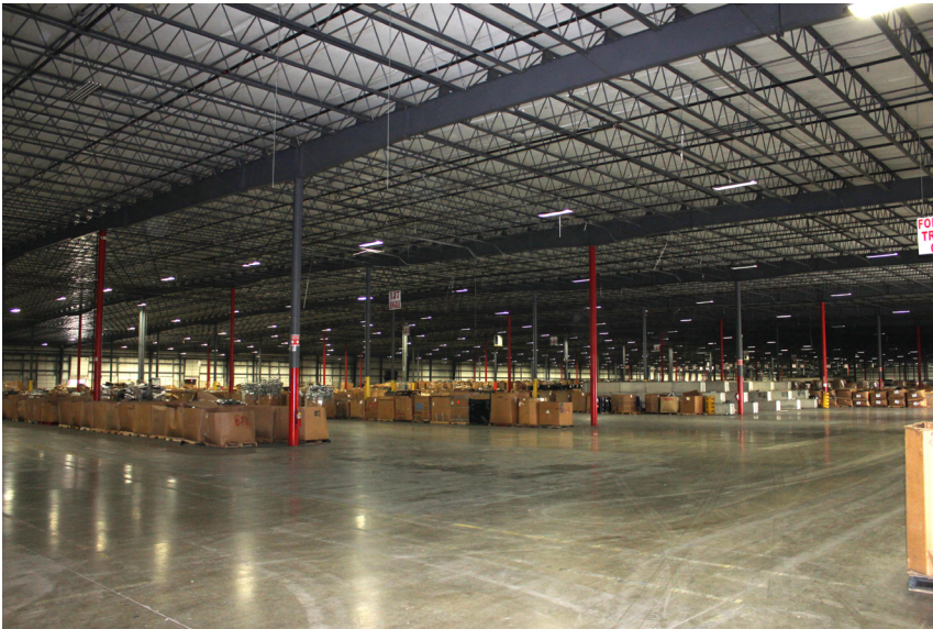
*Lighting recently upgraded to T-8 with motion sensors
